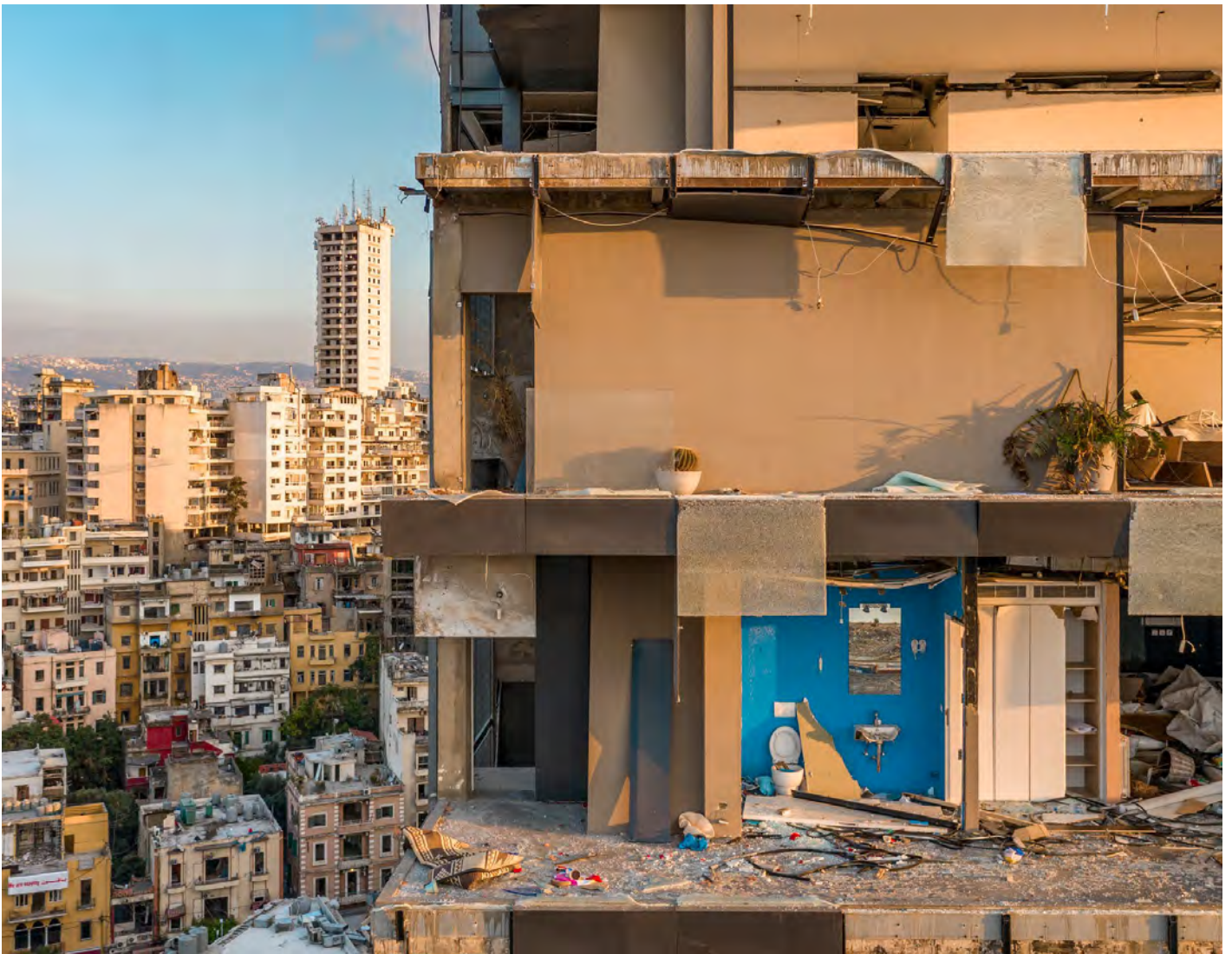
Destroyed architectural structures, post-blast. Credit: Rami Rizk
