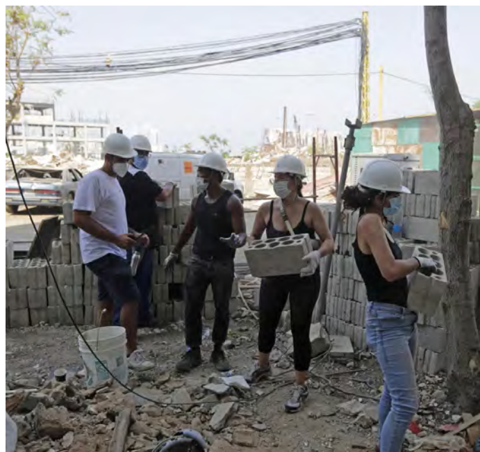
Volunteers help with the renovation of a Beirut flat belonging to an Armenian family. Credit: Anwar Amro
